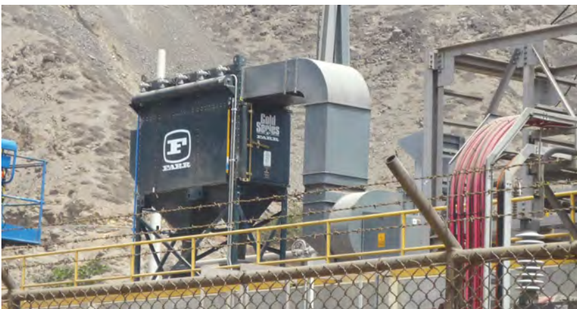
A 10-cartridge dust collector is installed on the roof of an MCC room to protect the equipment inside from dusty conditions of this South American copper mine. This equipment is operating above 4,000-m elevation.
