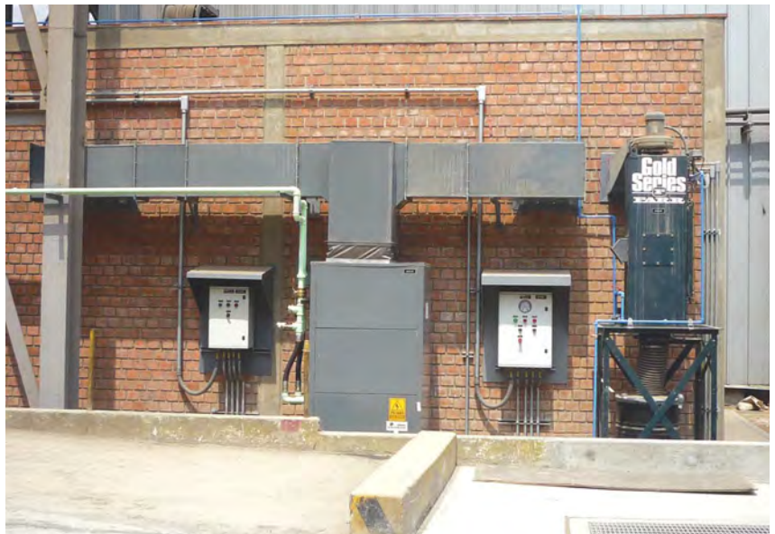
A small cartridge collector is used to pressurize an electrical room at a mine located in a warm climate. The dust collector is sized for 10% of the capacity of the electrical room's backpack-type A/C unit used for cooling.
