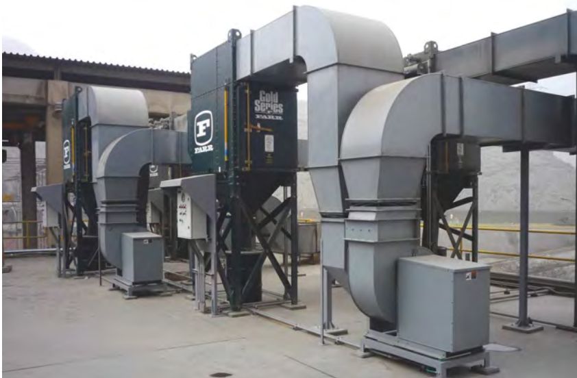
Multiple dust collectors, each containing six high-efficiency filter cartridges, are used to pressurize electrical rooms at a copper mine. The units have been operating for more than two years without a filter change. Blowers are controlled by VFDs and pressure sensors inside the room.
