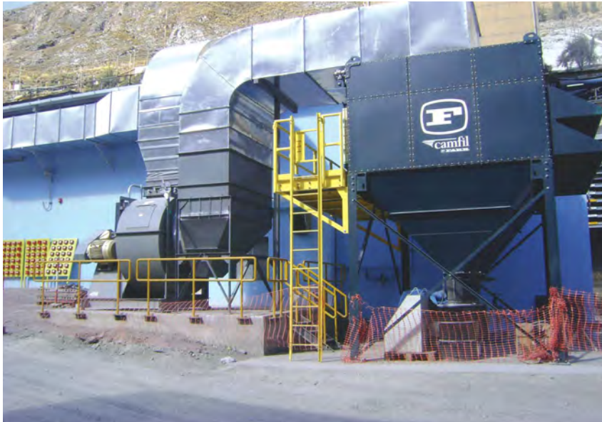
This 48-cartridge dust collector pressurizes and conditions the control room of a gold-silver mine located at an elevation of more than 15,000 ft (4,572 m).
