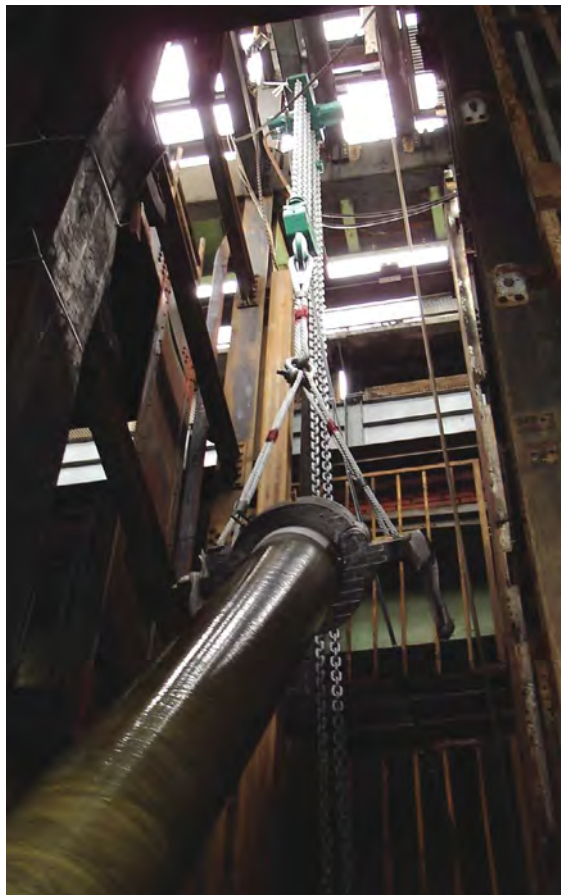
J D Neuhaus Profi 37 TI hoist handling a 1,000 m-long pipeline string weighing 30 mt, being positioned in a shaft.
