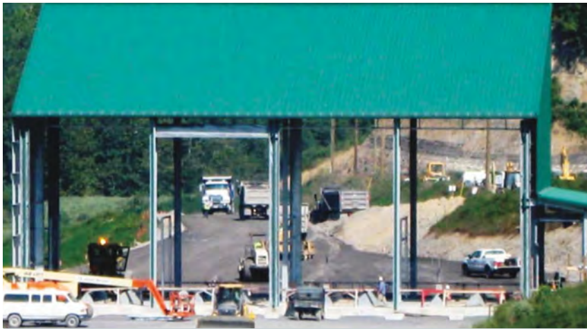
The truck dump facility has been designed for 400 trucks per day.
