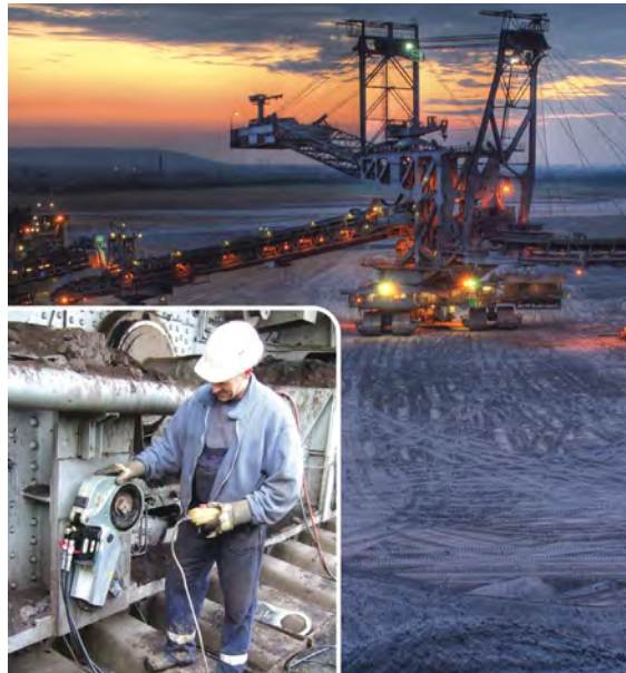
Getting the correct torque on critical bolts using a Plarad tensioning system.
