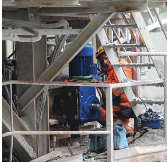
Nord's geared conveyor drives have helped NorStone improve plant availability.
